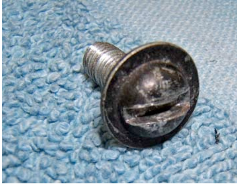
Screw with tethered washer before micro-scale application of black-pigmented anti-corrosion treatment (with a Sharpie).
